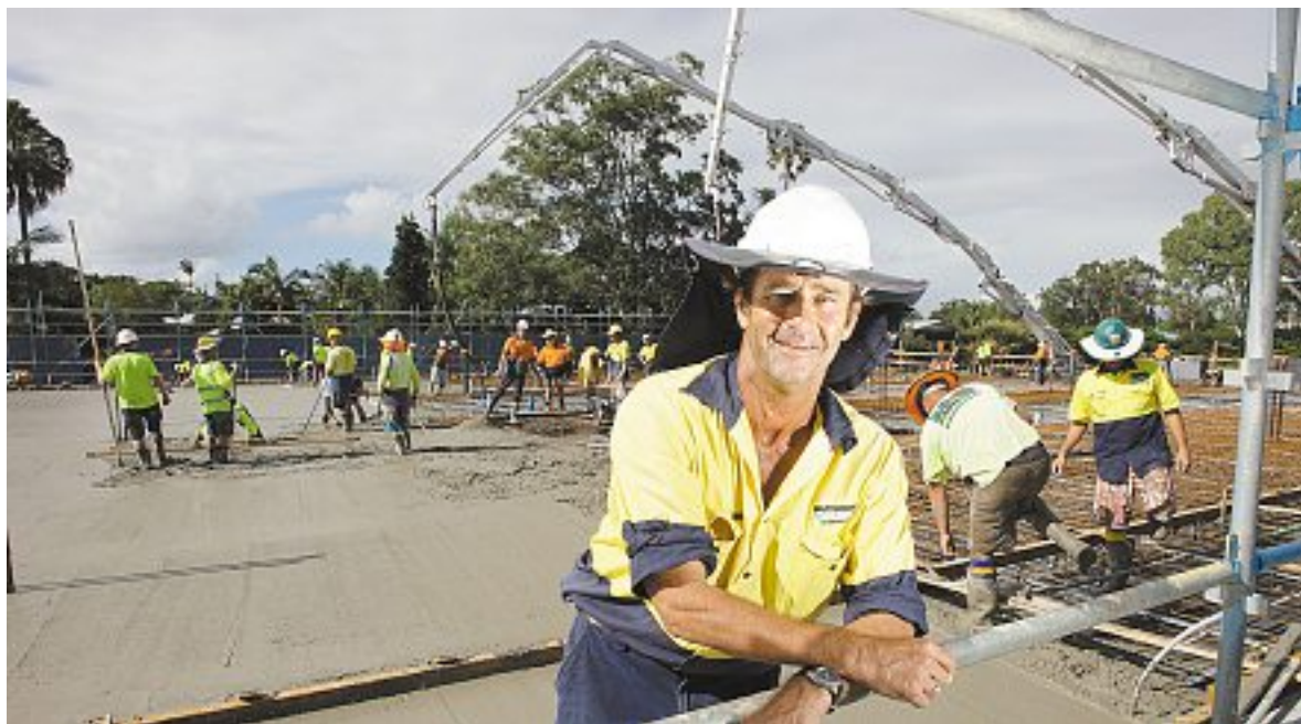
GOING UP: Hutchinson builders safety officer Lenny Thompson oversees the first-floor concreting for the Corporate Centre in Maroochydore.
